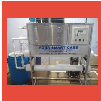
Reverse Osmosis Plant
