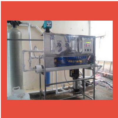
Reverse Osmosis System
