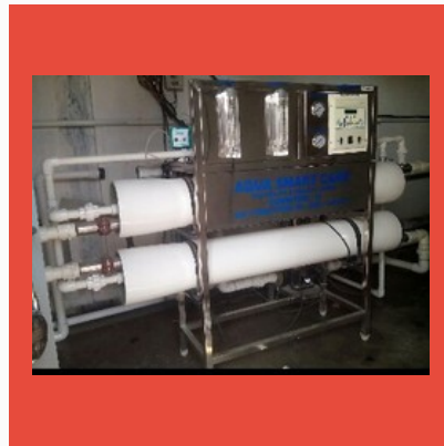
Commercial RO Plant
